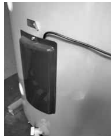
Figure 18 - Lower Tank Sensor
