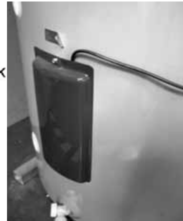
Figure 17 - Lower Tank Sensor
